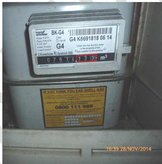
Gas meter reading
