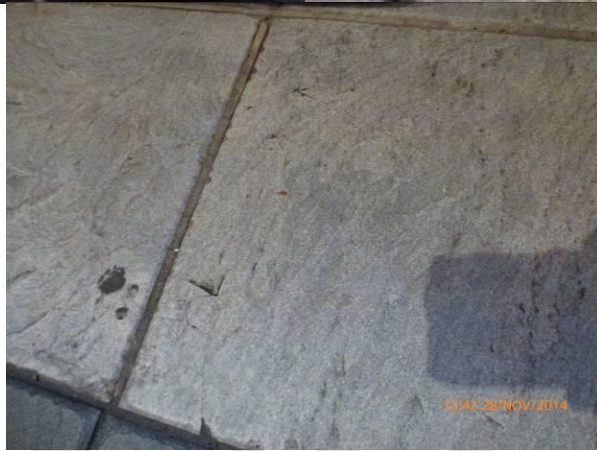
Item no.85 (various cracks)
